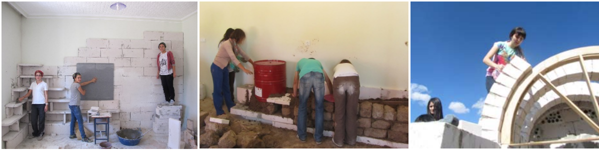
Figure 21. Insulation with AAC; rocket stove construction; building arch with AAC blocks during hands on course (2013).
