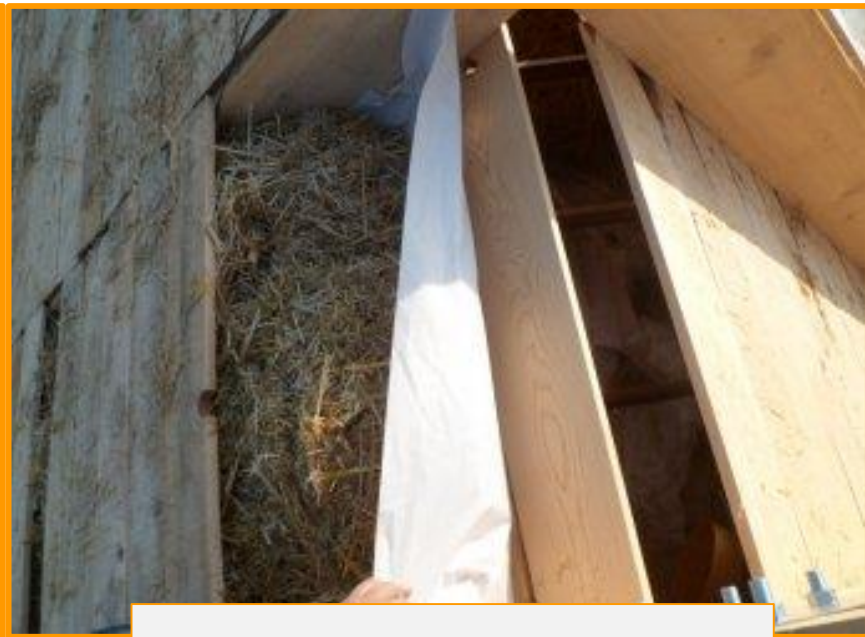
Loose straw between rafters
