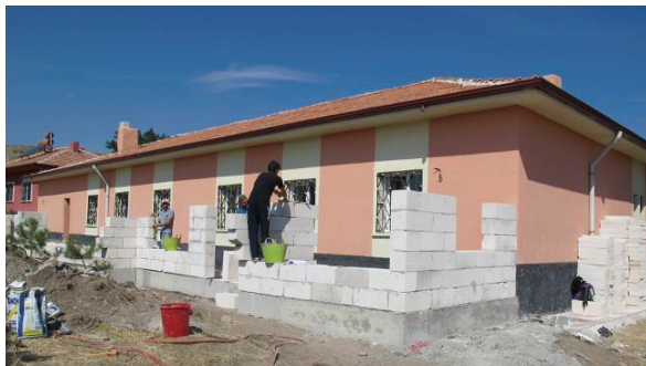
Fig 7: Building a solar space on the south facing side of the Sahmuratlı School.
