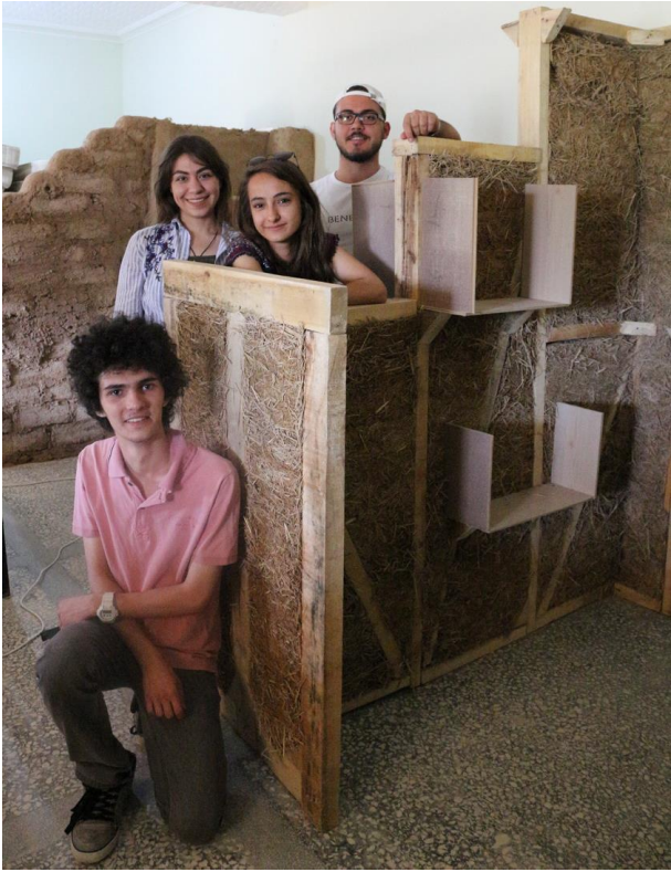
Figure 17. KTO University students built a new slip-straw partition wall in the dormitory. (17kekc0824)
