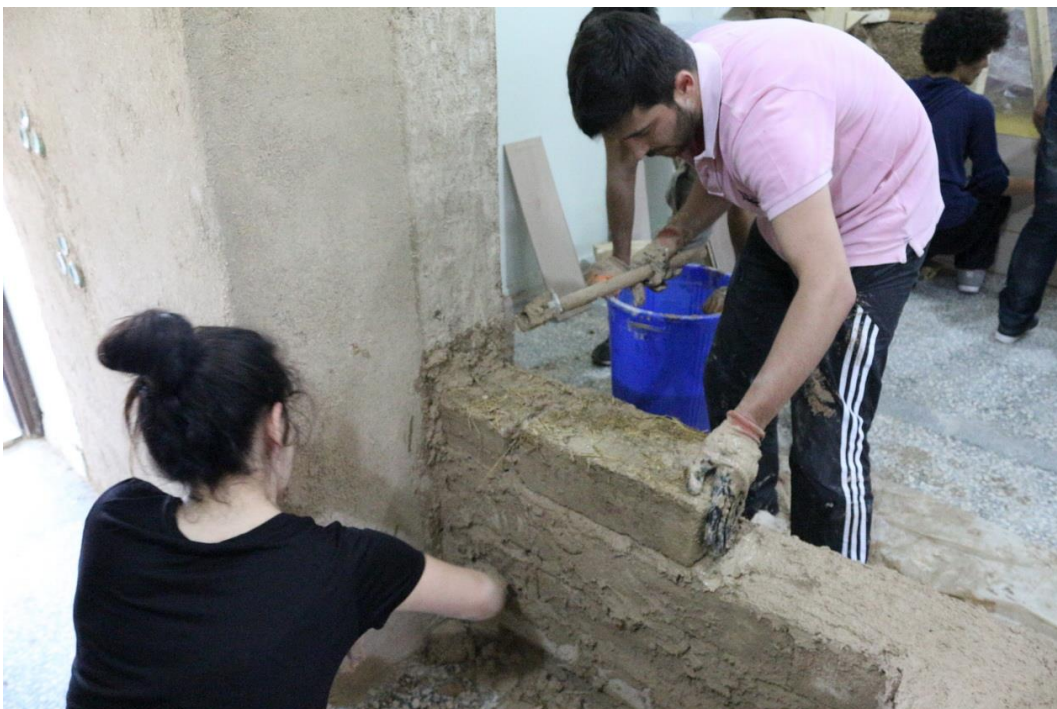
Figure 16. KTO-KÜ students making a partition wall with mudbricks in the dormitory. (17kekc0709)
