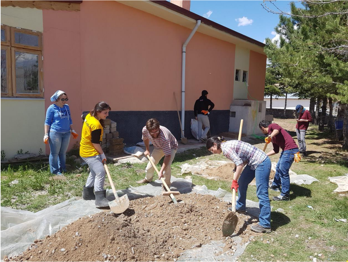
Figure 1. METU students preparing soil to make mudbrick during the Hands on session at Kerkenes in April 2017. (17kekc0406)
