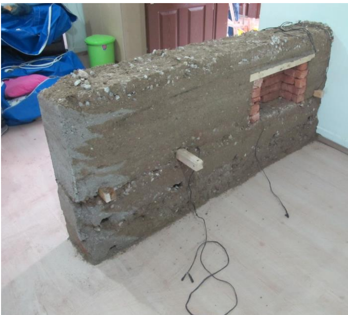
Figure 10. Rammed earth wall with a niche designed and built by METU students. (17kekc0247)
