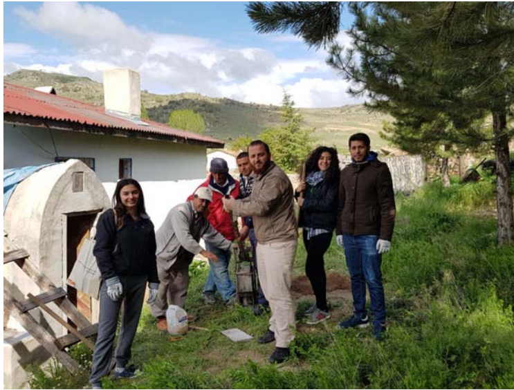
Figure 12. METU students making pressed bricks with the villagers during the Hands-on session at Kerkenes in April 2018. (18kekc0212)
