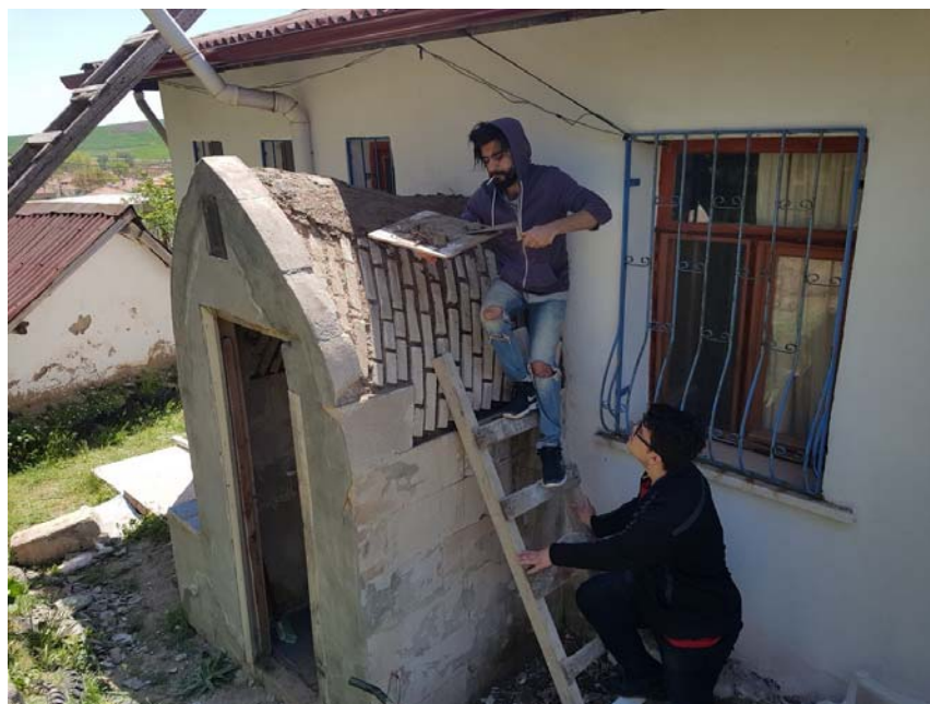
Figure 16. METU students plastering the AAC Nubian vault with the mud and oil mixture. (18kekc0253)
