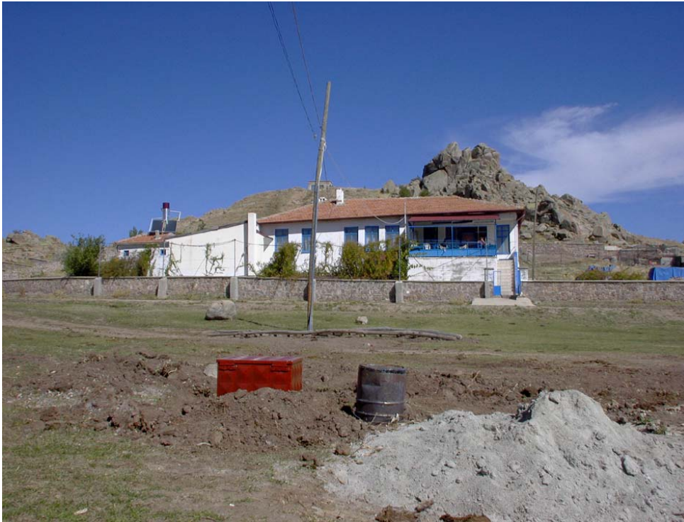
Figure 10: The pump was lowered into the drilled hole and a protective box placed on top. The electrical control panel is on the balcony of the Kerkenes House.
