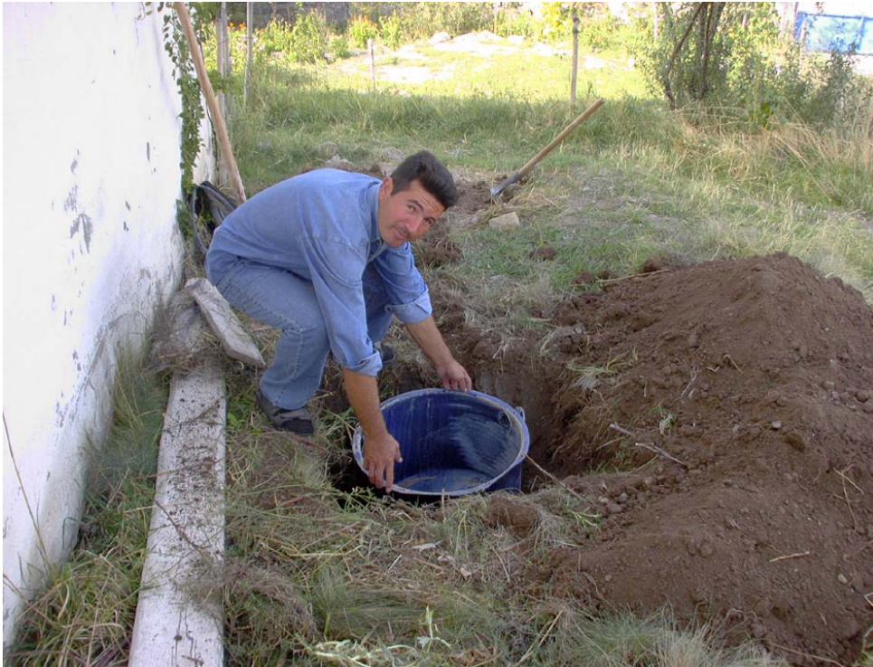
Figure 14: Settling tank, part of the old washing machine that caught fire, was lowered into the trench and connected to the bathroom plumbing.
