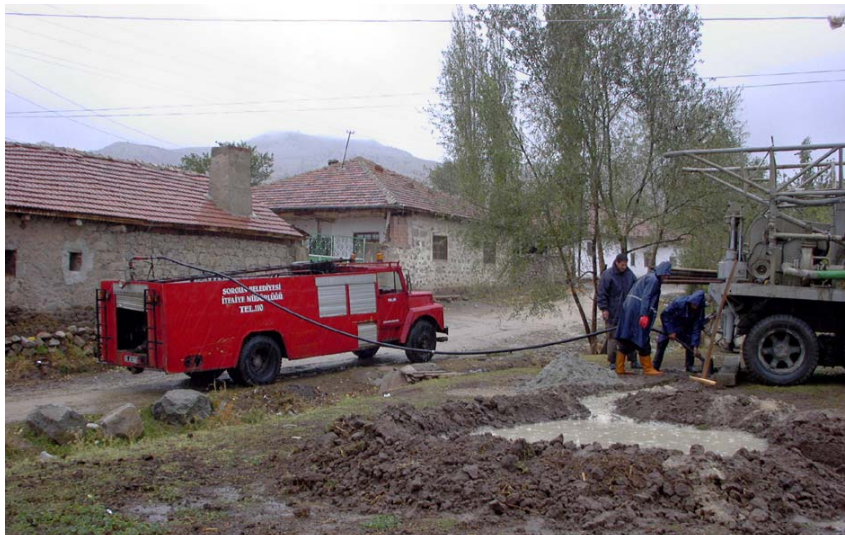
Figure 8: Any loose sand and small gravel needs to be washed out of the drilled hole so as to avoid clogging of the pump. The Sorgun fire Brigade willingly came to help us with that task!
