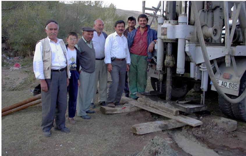
Figure 7: The drilling activities attracted our good neighbors, curious to see how much water would pour out. The drilling machine cored down to 17m into the granite, after which it was decided to stop.
