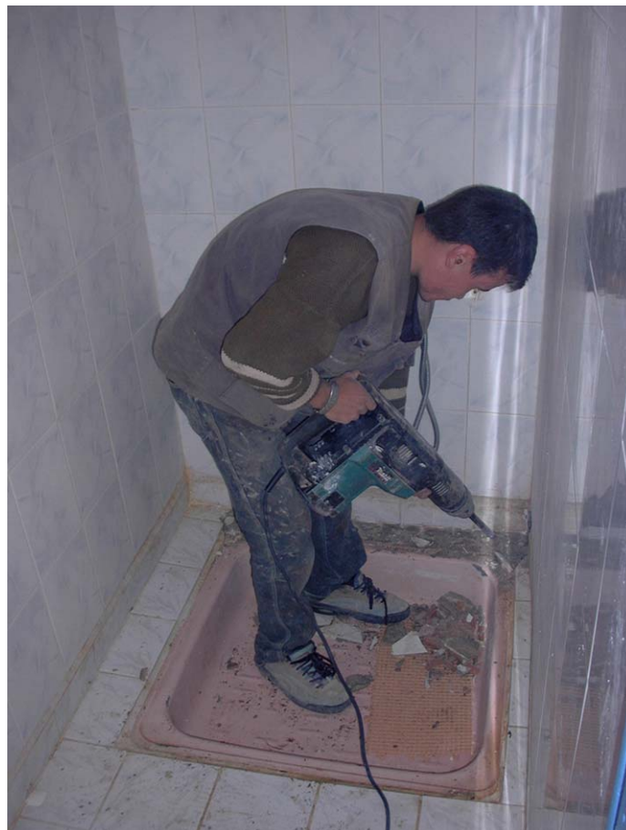
Figure 15: A new drain was added to the shower but the existing one kept so that a choice can be made if necessary.
