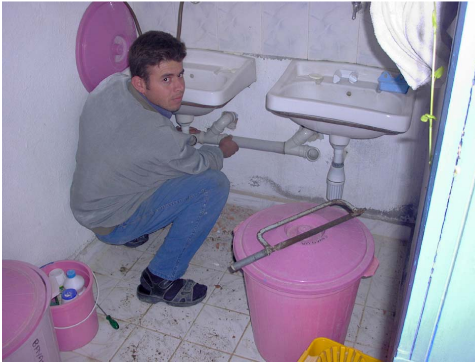
Figure 15: Plumbing in the bathrooms was altered to divert the shower and washbasin waste water to the grey water system.
