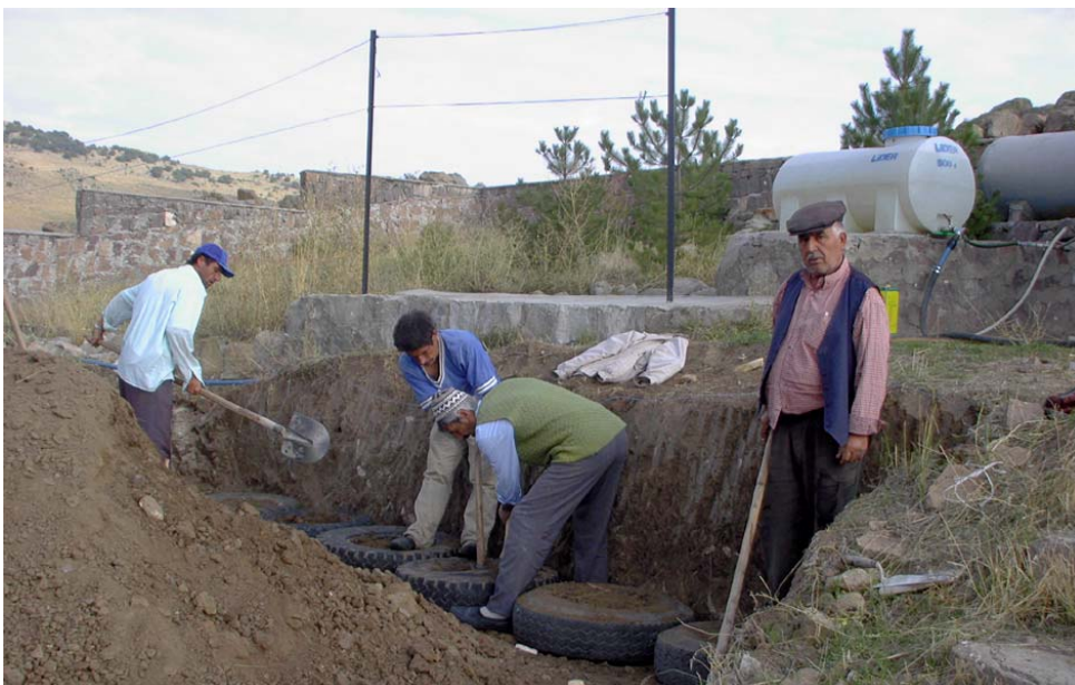
Figure 13: Old car tyres were used to build the retaining wall of the garden terraces. The water tanks used are seen on the level above.
