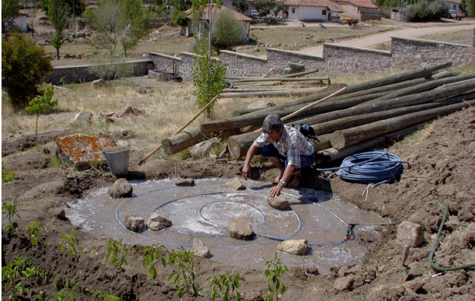
Figure 12: A perforated looped pipe is leveled, using a water cover, and then buried,
