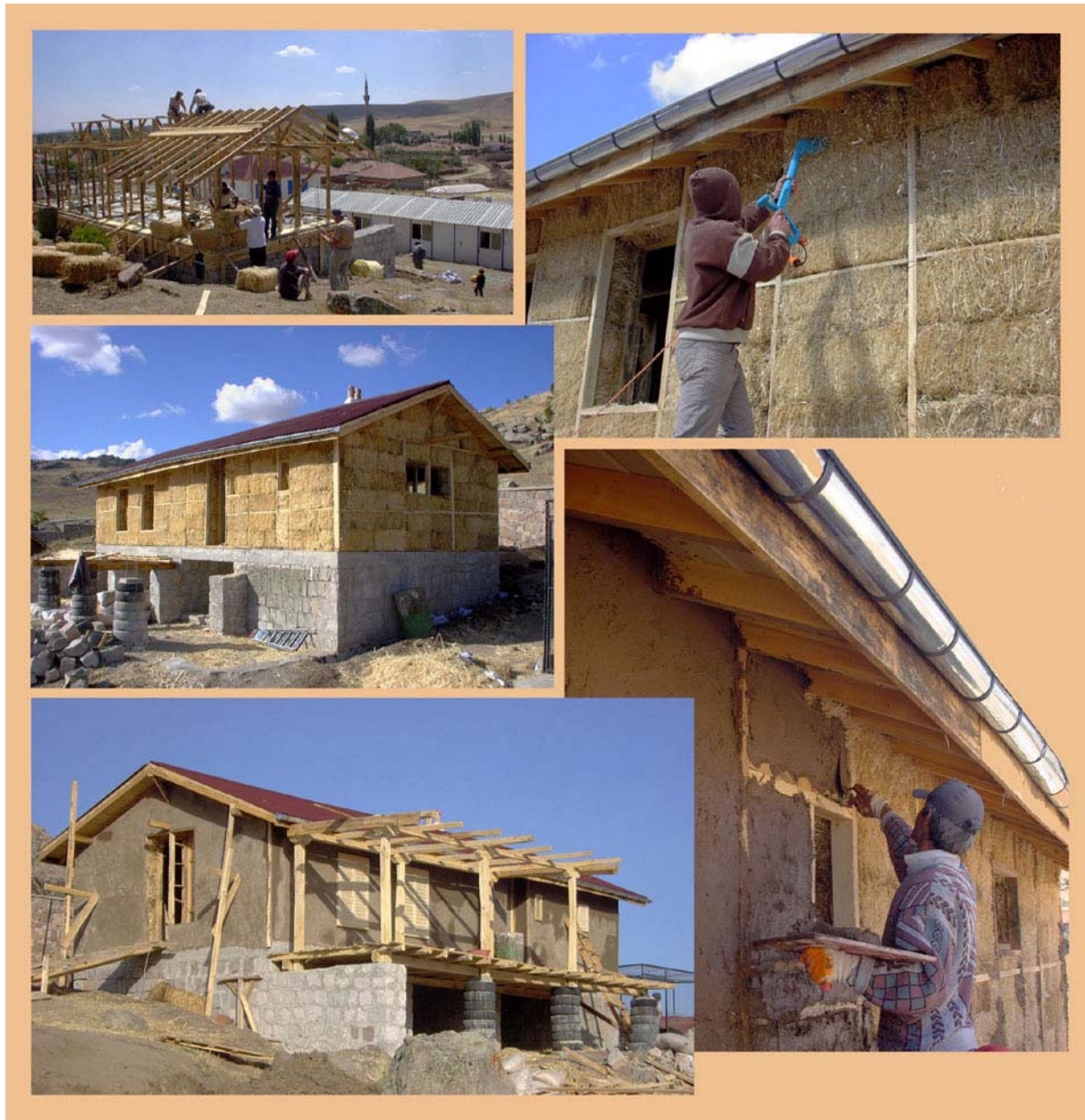
Figure 28. The straw bale house construction was well advanced by the end of September 2004. (04kejv0904, 04kejv1307, 04kejv1317, 04kejv1319, 04kejv1401)
