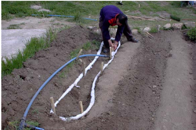
Figure 24. In the spring 2004 Memiş Gençarşlan set up a new experimental drip irrigation system, which uses geotextile wrapped up around the perforated pipes.
