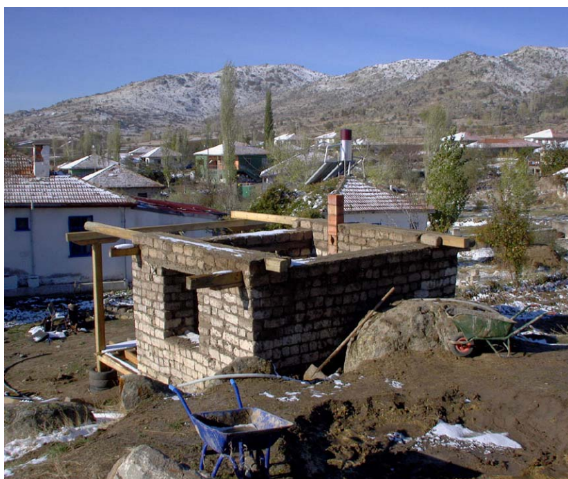
Figure 12. The new mudbrick building is designed to demonstrate the advantages of indigenous building materials and traditional techniques. (03kejv0504)
