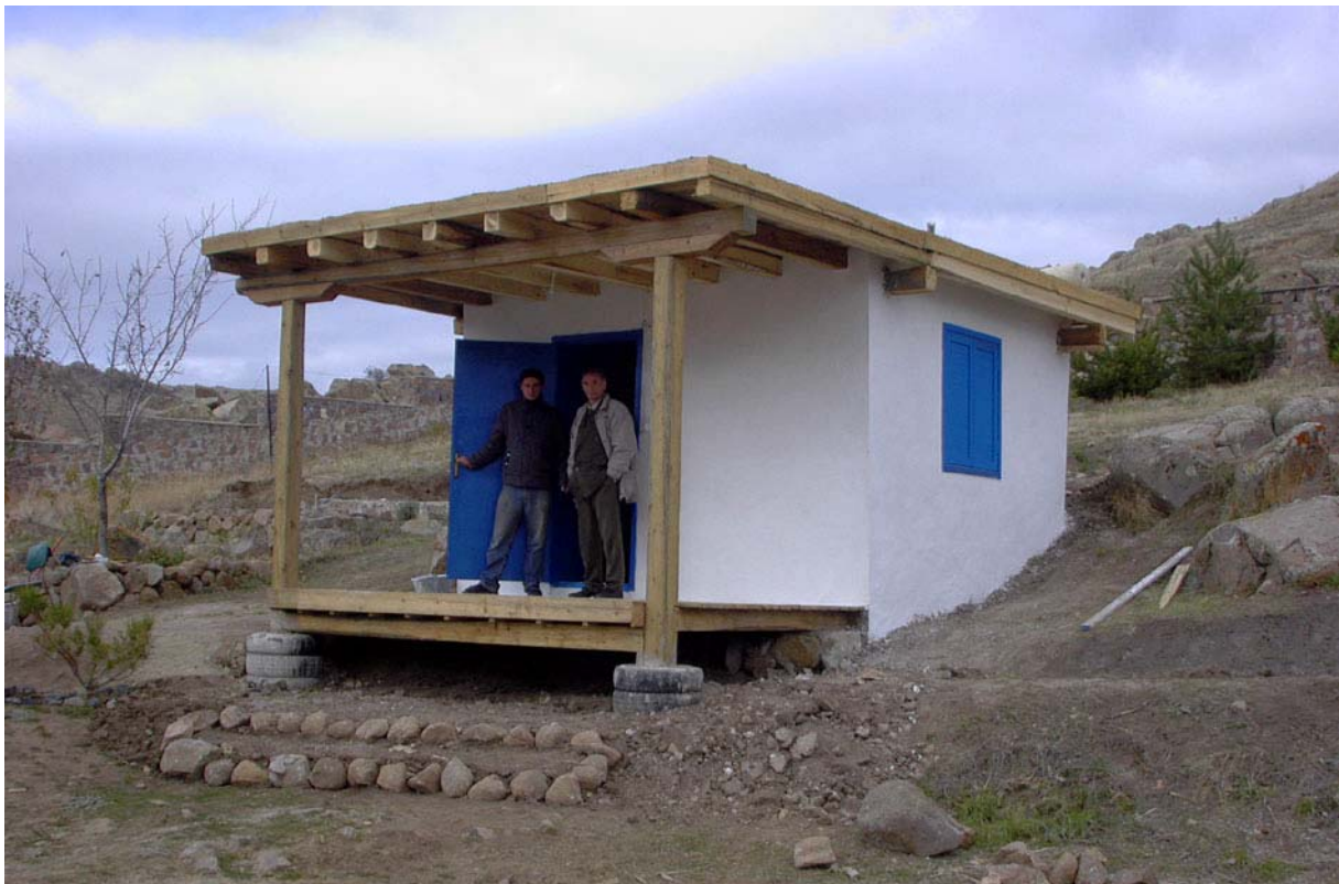
Figure 16. The new building will not only accommodate the Kerkenes Eco-Center but also be a model used for environmental studies. (03kejv0611)
