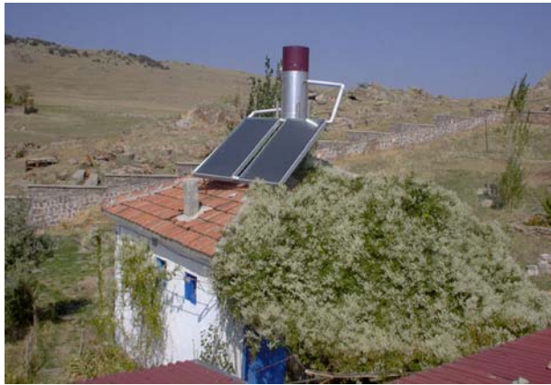
Figure 8. The solar water heater, used to provide hot water for the showers, proved to be very efficient and economical. (03kejv0408)
