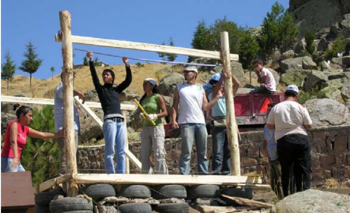
Figure 22. During the 'Hands On' activities at the Kerkenes Eco-Center, METU architecture students and villagers built a shelter for the solar driers. (08kenc1213)
