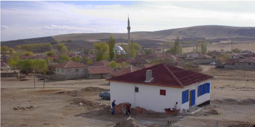
Figure 3: The last finishing touches are added to the new storage and laboratory building.
