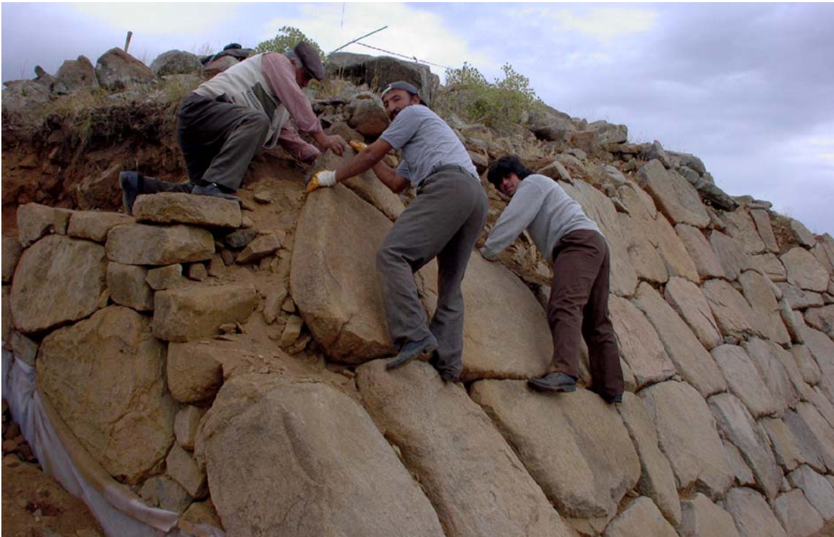
Figure 47: Some of the stones in the glacis were reset in their original positions to prevent them falling during the winter. The passage itself was lined with geotextile and covered with rubble in order to protect the original surface. (02dpjv5610)
