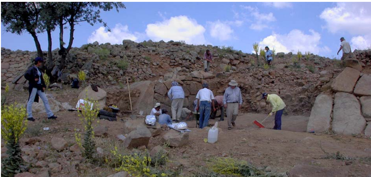
Figure 44: When the entire gate passage has been cleared and a new protective surface laid, visitors will be able to enter the city through the original gate. (02dpjv2204)
