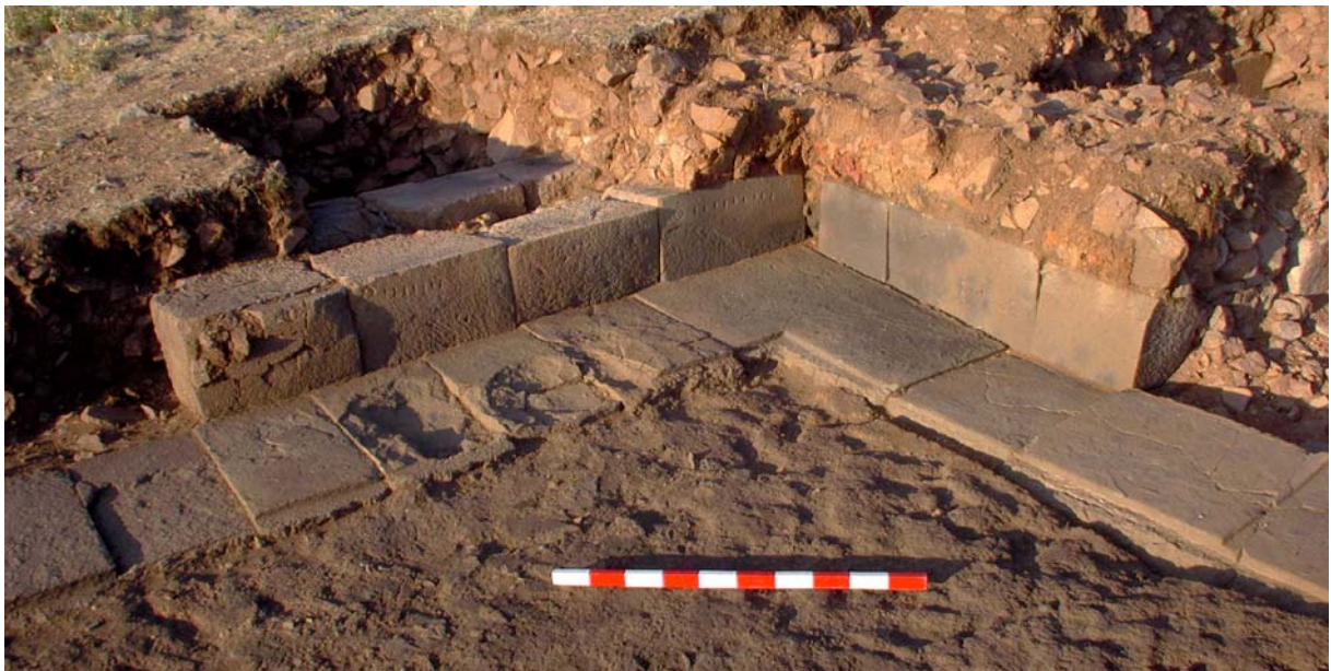
Figure 37: The intense heat of the fire damaged the granite ashlars as well as the sandstone pavers. The upper walling comprised rubble filling a timber frame coated with mud plaster. (02dpjv3609)
