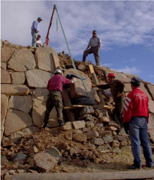
Figure 79. Using a winch to replace large stones that had fallen from the face of the glacis. Ministry Representative Mehmet Katkat skilfully supervised this operation. (03dpjv5616)
