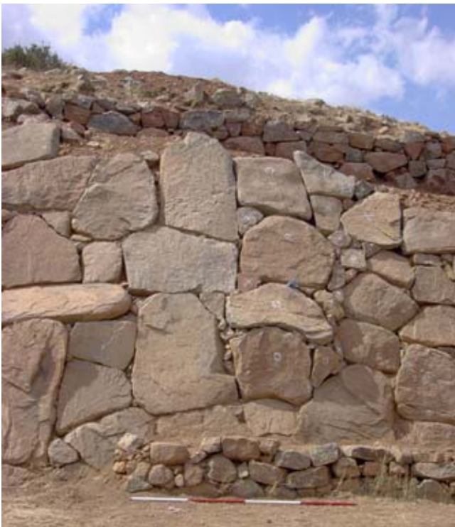
Figure 80. The glacis and the tower wall behind after conservation. A full record was made of which stones had been replaced and which were newly introduced. (03dpjv6753)
