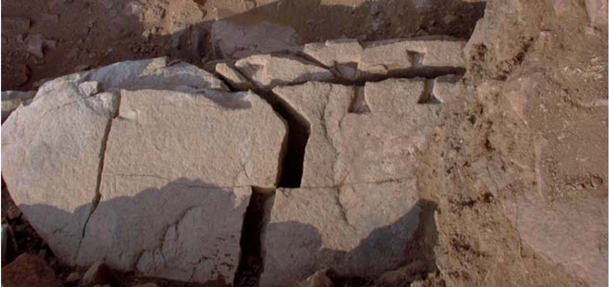
Figure 18. A row of small clamp cuttings for mending the front of a split granite block in the north wall of the South Tower. This is probably a corner stone, the end being just beyond the baulk at right. (04dpjv2219)
