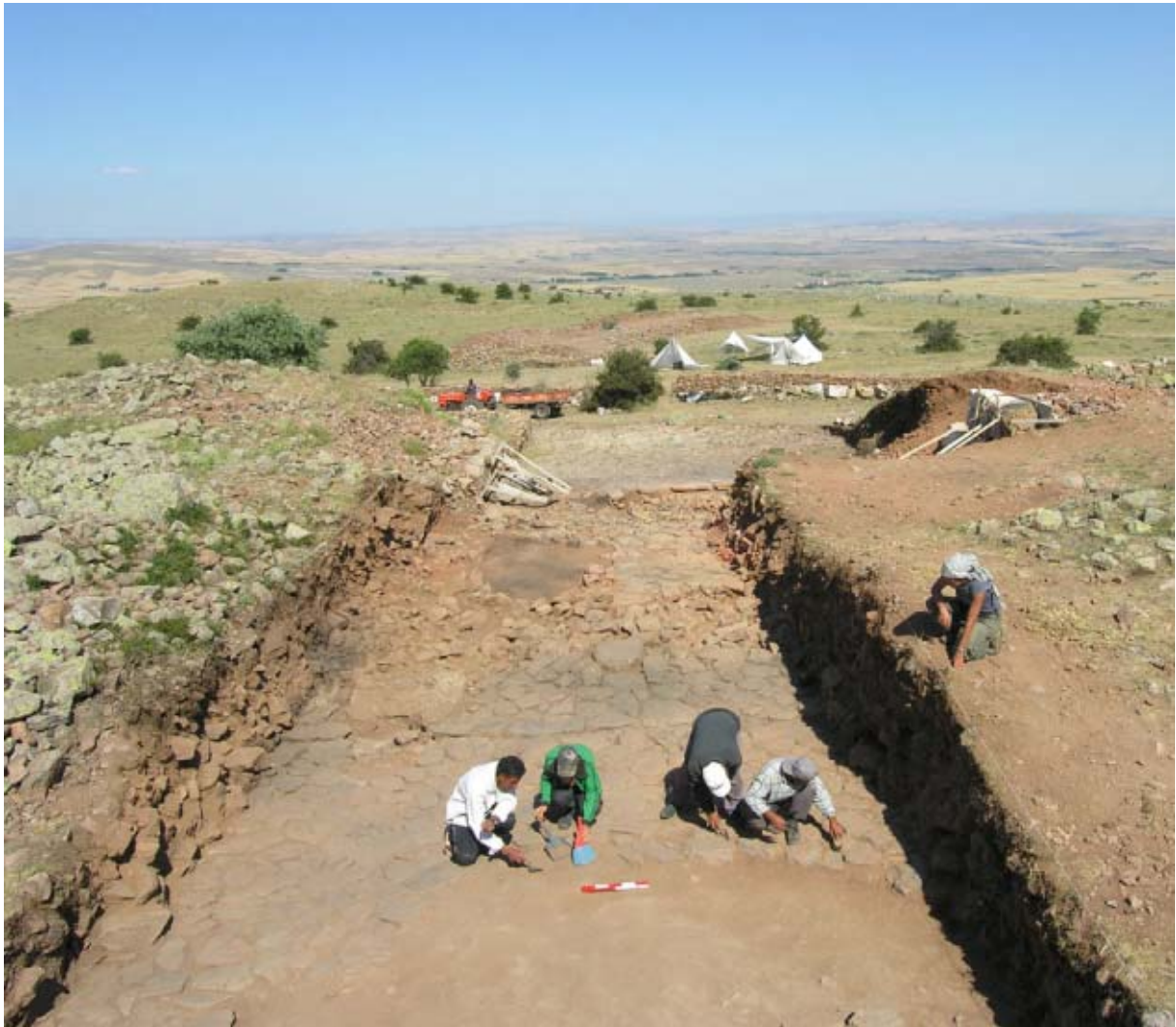
Figure 9. Excavation of the Monumental Entrance to the Palace Complex, looking east down the passageway between the two towers. Temporary wooden shoring supported the structurally unstable walls at the front end of these massive towers. Workmen are brushing the western stretch of stone pavement extending beyond the rear façade of the monument towards the Audience Hall. (05dpnc0155)
