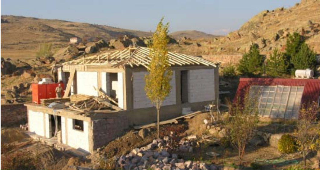
Figure 5. Construction of the Erdoğan Akdağ Center for Research and Education. AAC blocks, cement, sand and roofing sheets were donated by AKG Gazbeton, YL Yozgat Çimento, the Sorgun Belediye and Onduline respectively. (05kenc0628)
