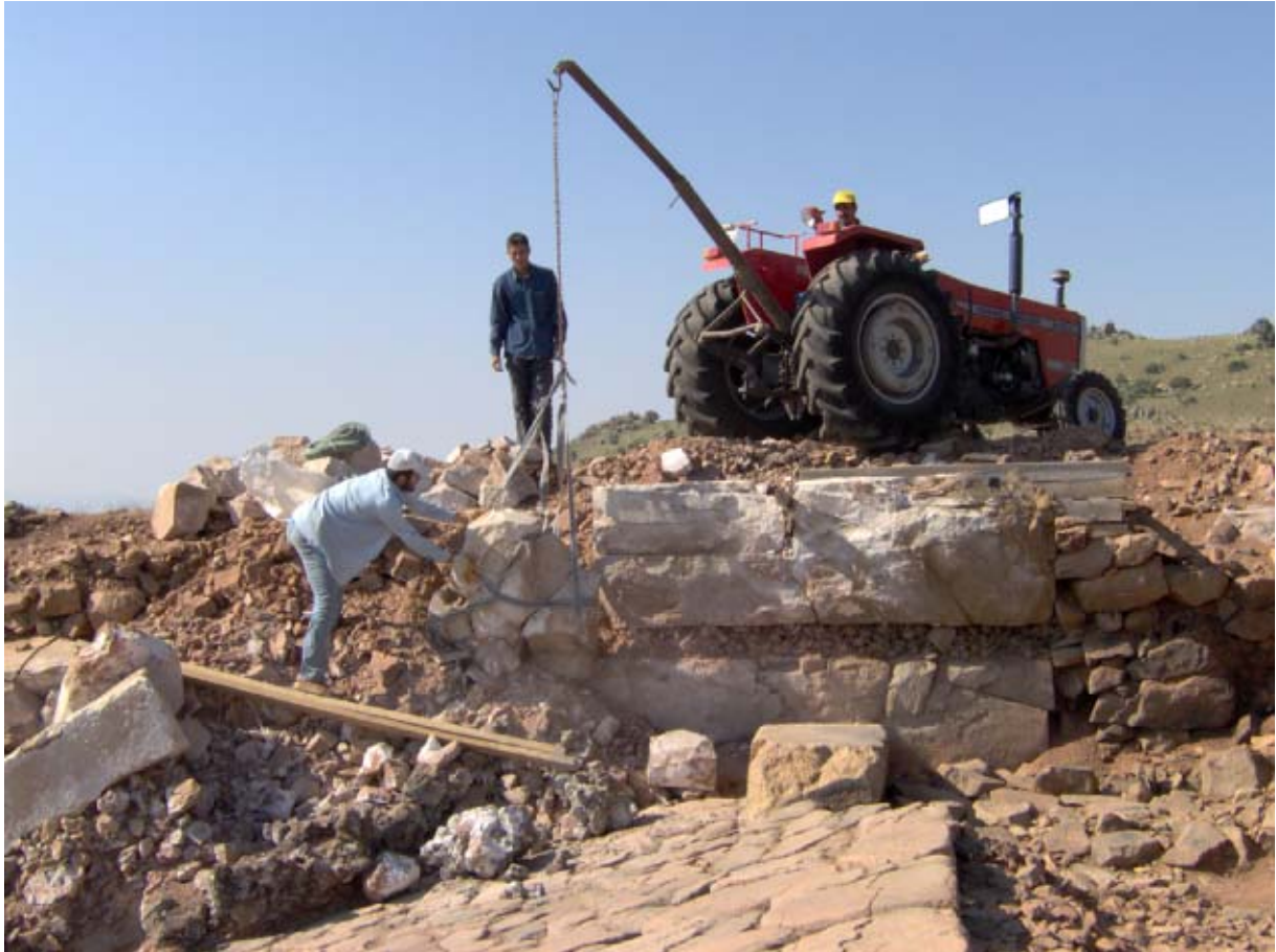
Figure 24. The horizontal gap left between courses after the horizontal beam completely burnt down caused the wall of the South Tower to become structurally unstable. Facing blocks and burnt debris are naturally coated with white carbonates. Many of the large stones, shattered by the intensity of the fire, had to be removed for safety. (05dphp1104)
