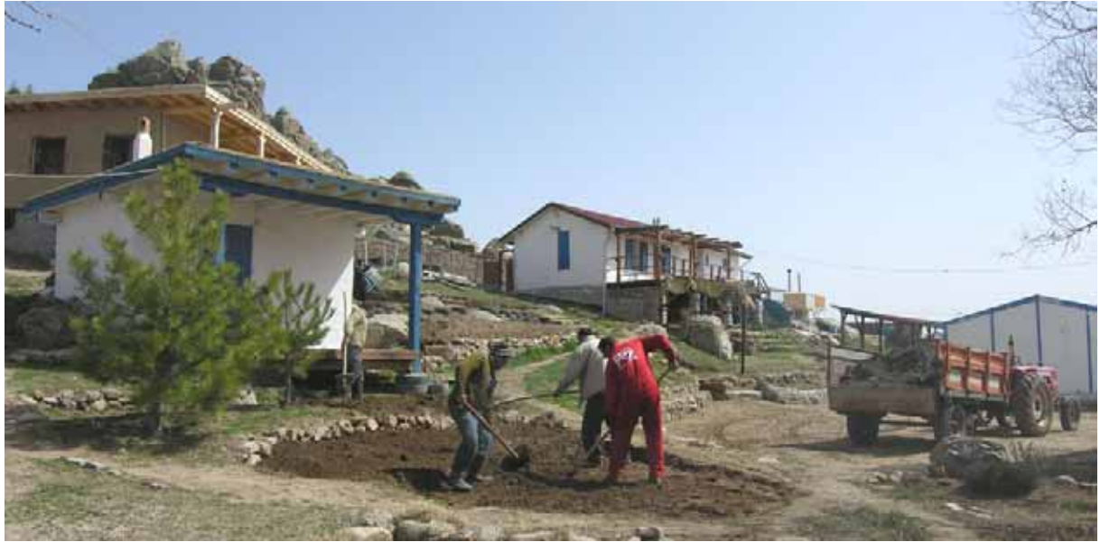
Figure 12. Between the mudbrick workshop, at left, the strawbale house, at centre, and the four-room prefabricated building, at right, the garden is being prepared for a good crop of organically grown vegetables. (07dpnc0216)
