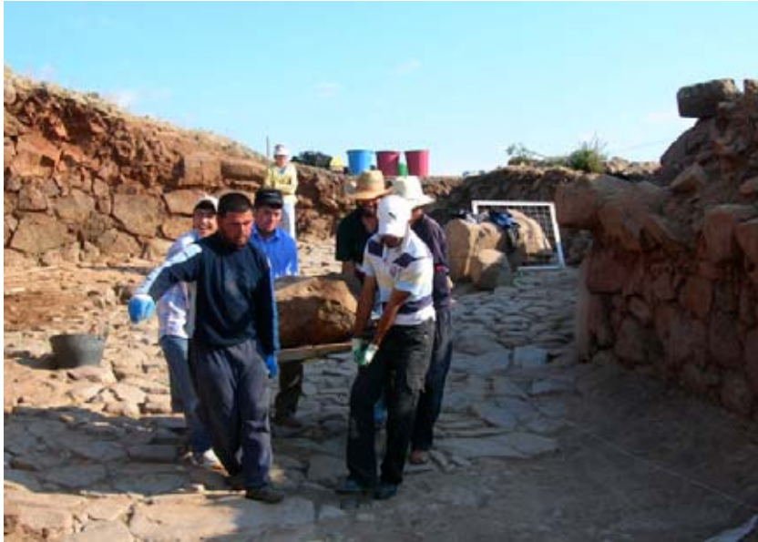
Figure 27. With no access for machinery big blocks are moved by manpower. (09dpng2806)
