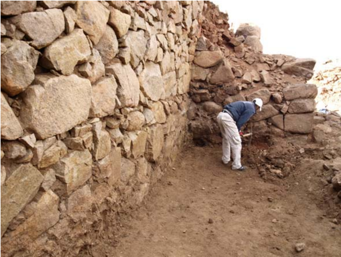
Figure 107. The level of horizontal timbers in adjacent walls do not always coincide. (10dpkc2253)
