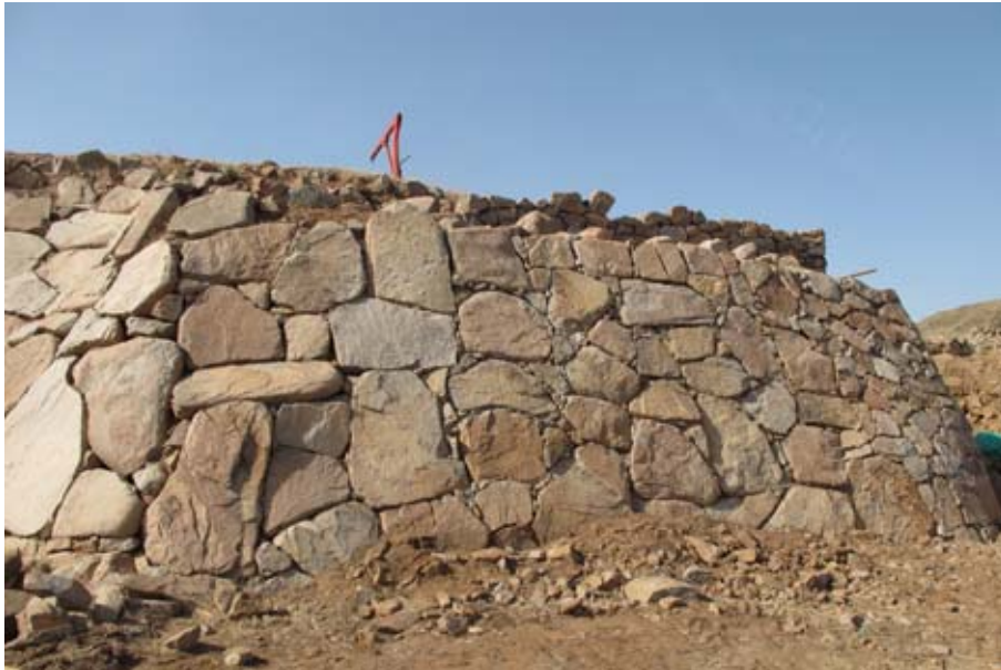
Figure 143. Once the east side of the glacis was built up to the height of the adjacent stretch of glacis, it was found necessary to relocate two slipped stones, at left, before rebuilding the top of the glacis. (10dpcg0318)
