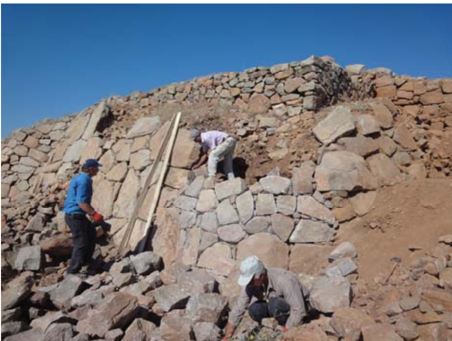
Figure 140. The east corner was restored before the remaining portion of the glacis was uncovered, thus providing structural stability and minimising the risk of further collapse. (10dpkc3302)
