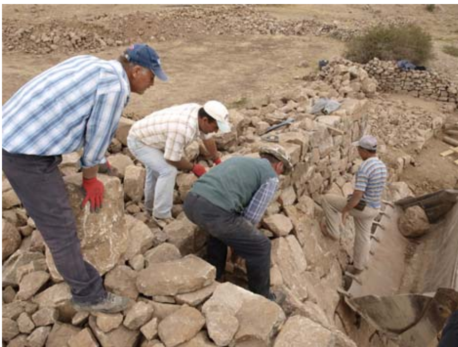
Figure 133. Once the East Tower wall was safely built up, it was possible to raise the large city wall on top of its existing base. (10dpkc2505)
