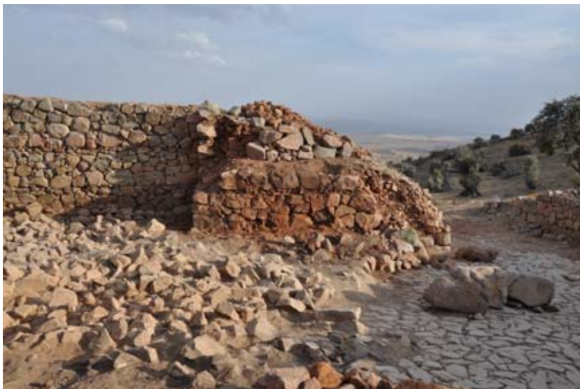
Figure 99. The wall's lack of structural stability is a result of the gap left by the horizontal timber beam after it burnt out. (10dpnd1390)
