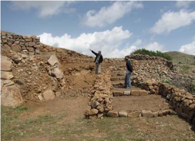
Figure 137. Temporary access was created in the spring to facilitate excavation work at the junction of the East Tower and the City Wall. (10dpcp0913)
