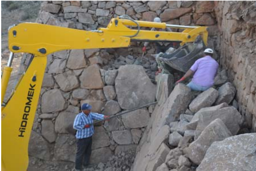
Figure 150. The machine's bucket was used to lift large and heavy stones. (10dpnd1395)
