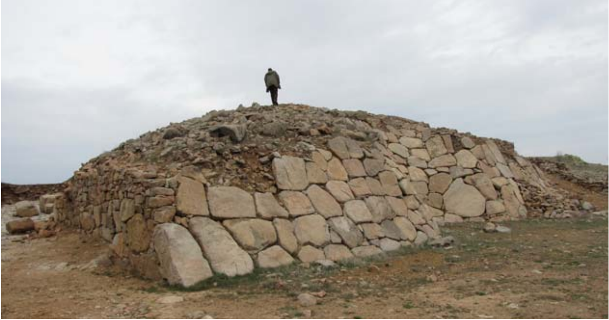
Figure 126. The Cappadocia Gate glacis photographed in May 2010 before the start of restoration work. (10dpcp0118)
