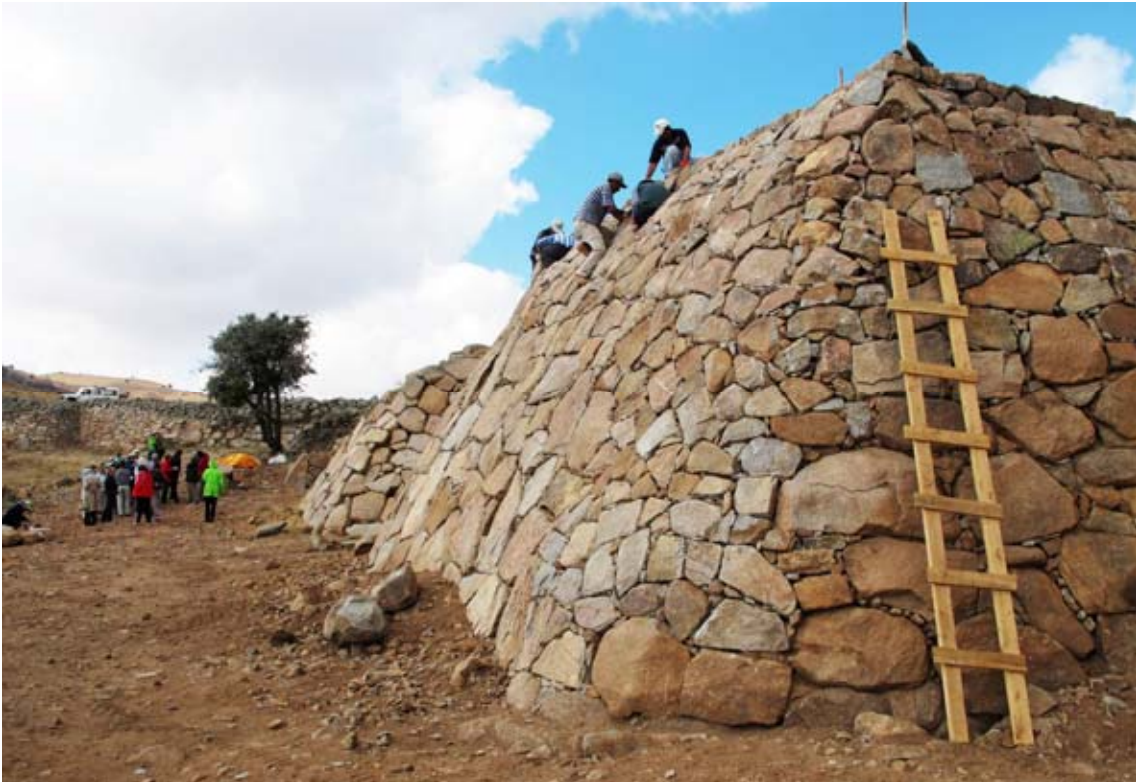
Figure 131. The restored glacis looking west. Visitors are standing in front of the 6m wide passage. (10dpcg0601)
