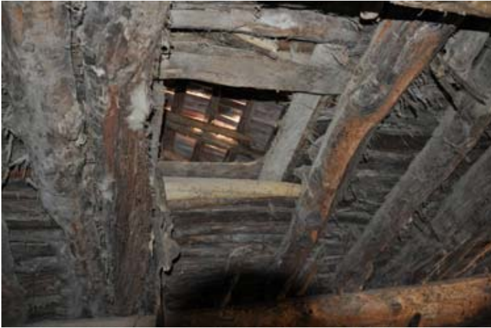
Figure 65. The original flat roof was constructed of beams supporting rafters covered with split branches and a thick layer of mud. A trap door cut through the original roof provides a glimpse of the recently added clay tile pitched roof. (10dpnd1905)
