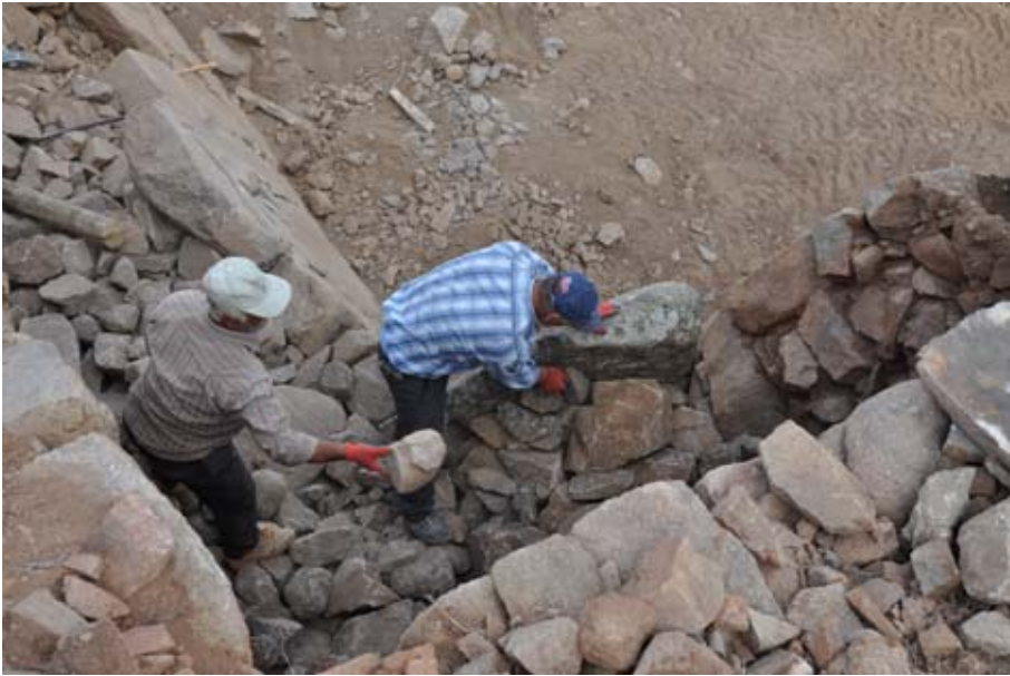
Figure 152. Small and medium stones were selected to fill up the space behind the facing stone. (10dpnd1387)
