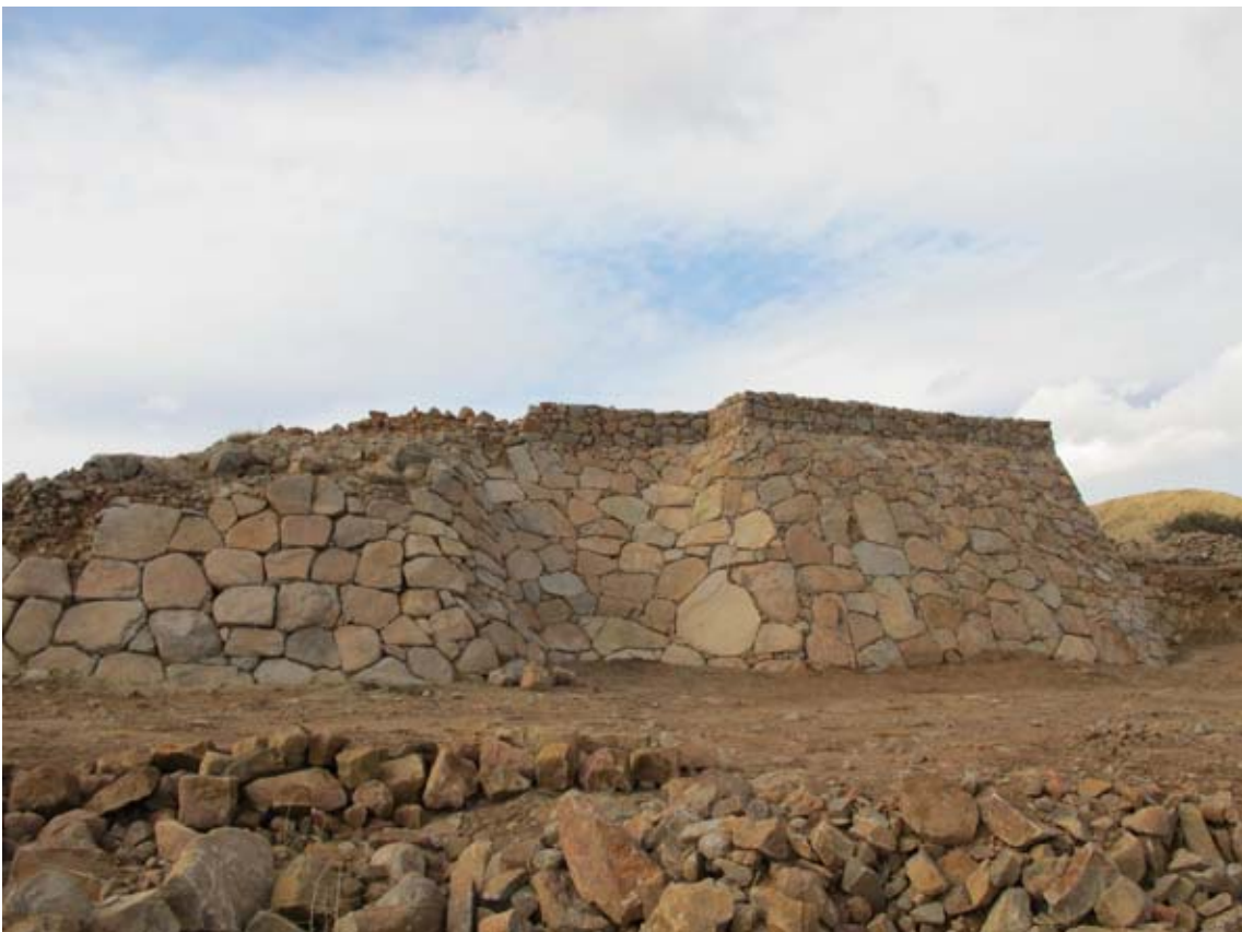
Figure 132. The Cappadocia Gate glacis at the end of the 2010 restoration campaign. (10dpcg0935)
