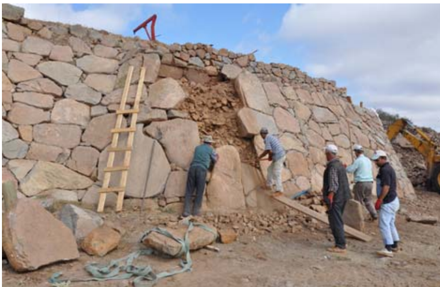
Figure 144. The machine operator skilfully lifted the upper stones to bring them down. The large stone that had slipped forward was pushed back in line with the glacis face. (10dpnd0848)
