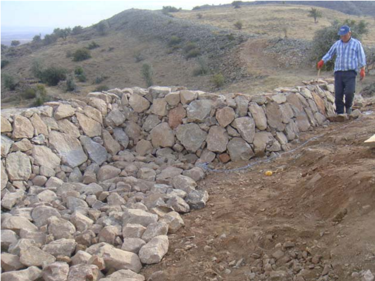
Figure 155. As a safety measure, the restored tower walls have been raised to form a parapet preventing visitors from walking too near the edge. (10dpkc3942)
