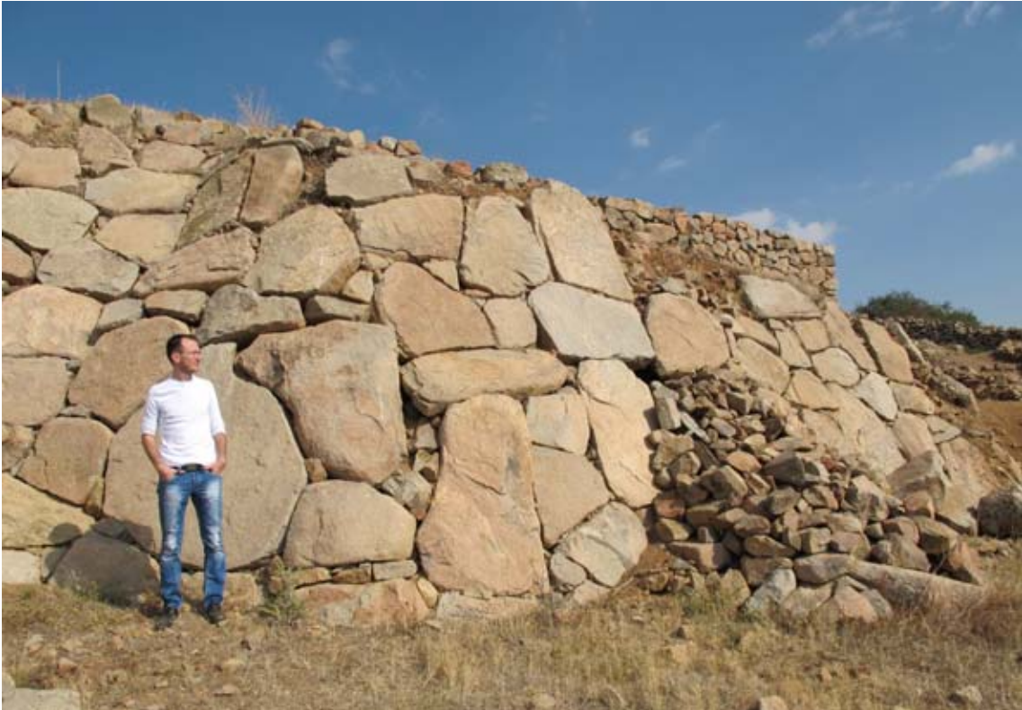
Figure 134. Architect Erkan Kambek contemplating the huge task ahead before the restoration work started. (10dpcg0232)
