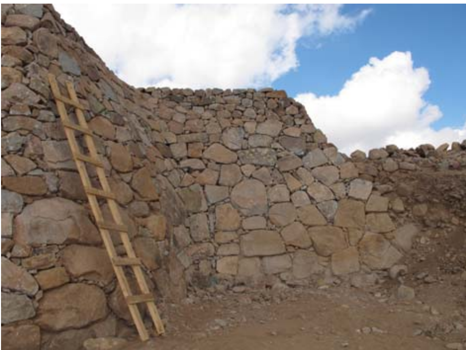
Figure 154. The junction between the East Tower and the massive defensive wall. (10dpcg0610)
