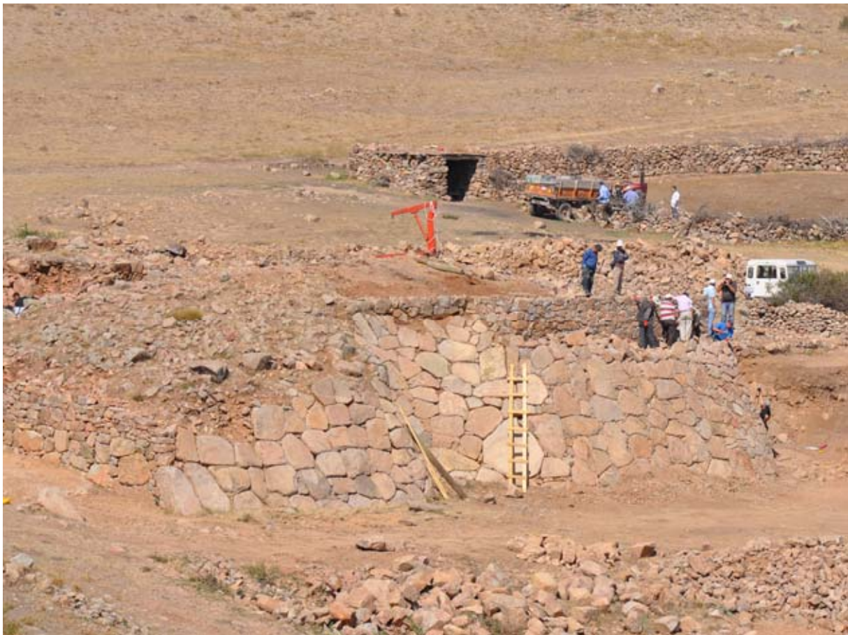
Figure 130. Stones, previously cleared from around the Gate structure and dumped nearby, were used to restore the glacis. (10dpnd1121)
