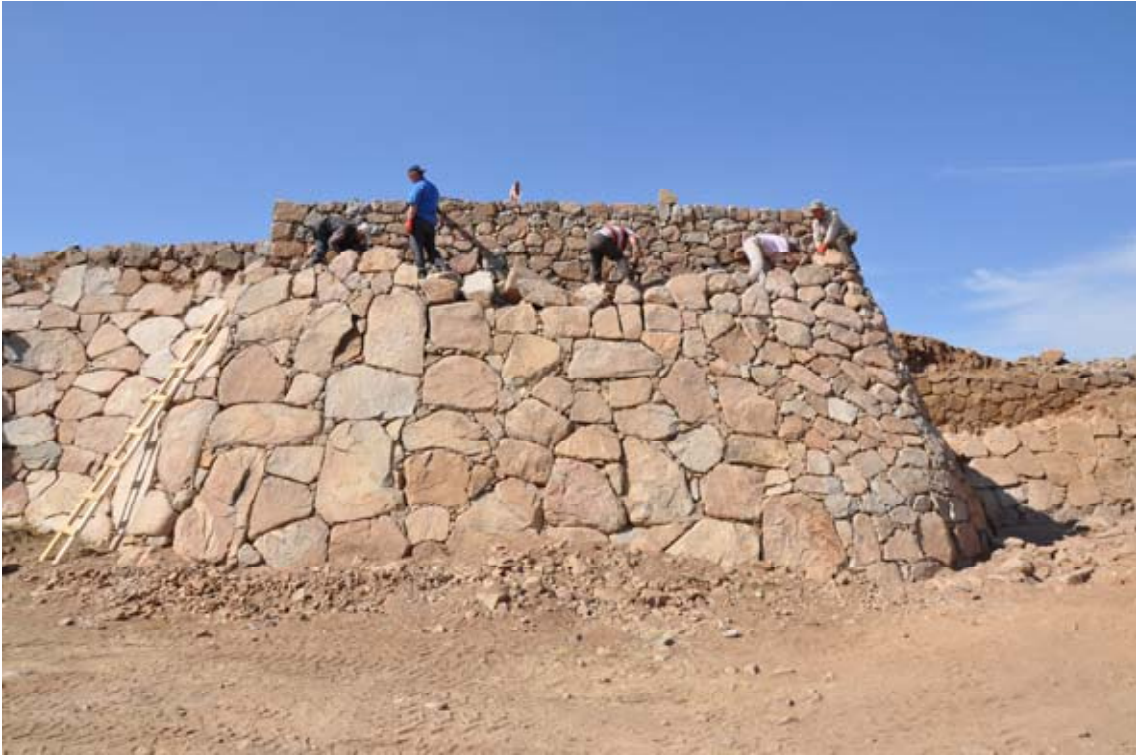
Figure 148. Once the two large stones in front of the Middle Tower were moved back to their original position it was possible to rebuild the glacis to its original height. (10dpnd1141)
