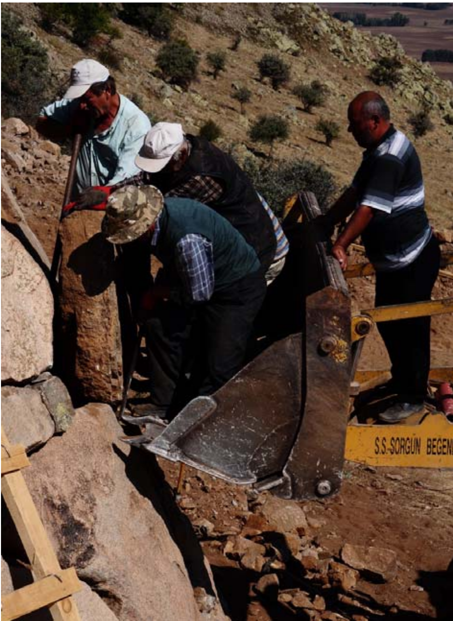
Figure 147. Stones were lifted up and pushed back into their original position. (10dpnd0882)
