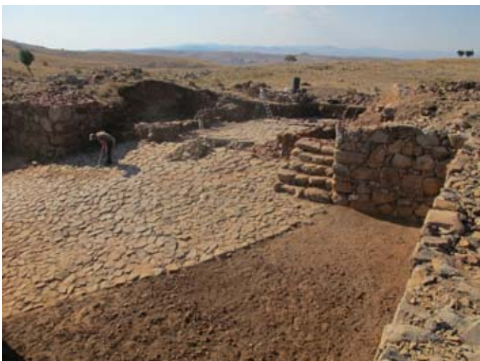
Figure 80. Final stages of cleaning the extensive stone pavement after repair of the West and East Towers. (11dpcg3029)
