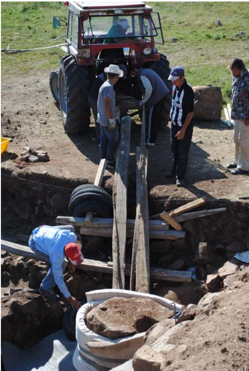
Figure 68. The core of the plinth was pulled out of the trench by the tractor. (11dpkc1928)
