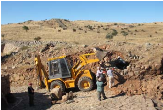
Figure 78. Very large stones that had fallen onto the pavement from the tower corner could only be moved by more powerful machinery. (11dpcg2412)
