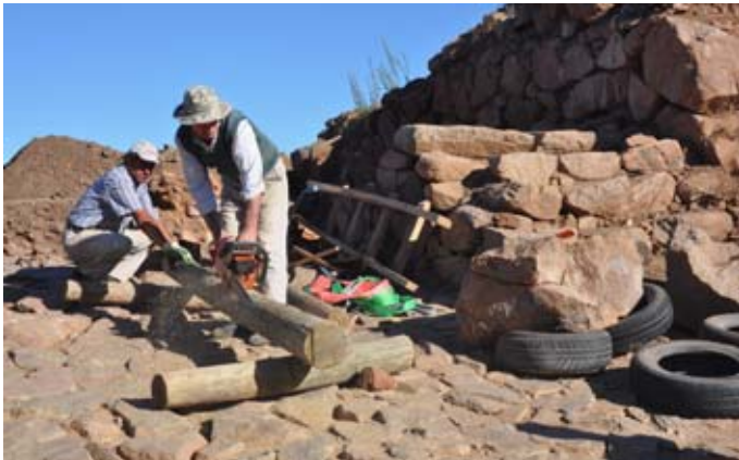
Figure 75. Secondhand telephone posts were squared off before incorporation in the restored wall. (11dpnd2356)
