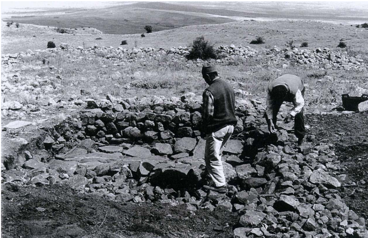
Figure 7. Back-filling TT17: the base and sides of the trench were marked with nylon rope and strips of plastic. Broken glass was placed on original wall tops which were then capped with new stone.
