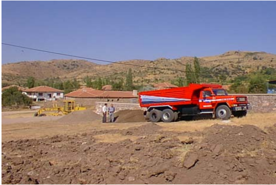
Foundations for the newbuilding were started in August 2000 but it was decided to resume the construction in spring 2001.
