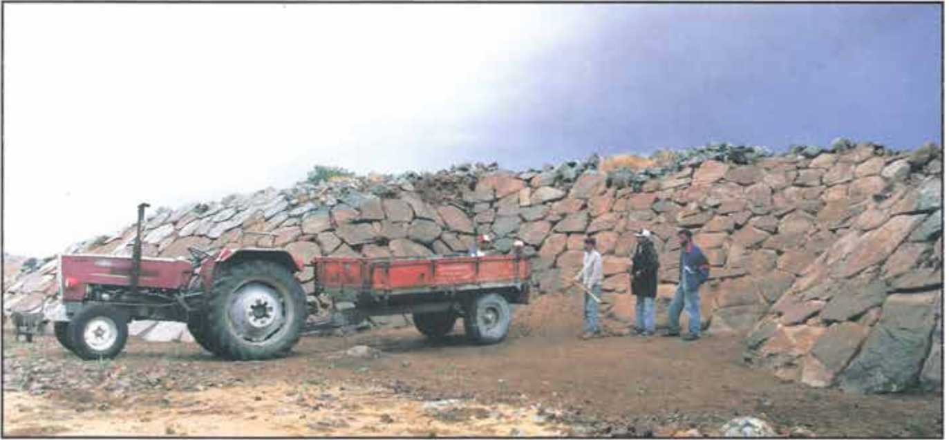
Figure 12: At the end of the season a protective covering of clean sand and gravel was laid over the base of the "Palace Complex" façade. Trials are being made to see if geotextile will inhibit plant growth and deter burrowing rodents.
