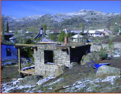
Figure 18: The new experimental unit using a traditional timber frame and mud-brick walling on stone foundations with a flat mud roof under construction. Kerkenes Dađ dominates the horizon.
