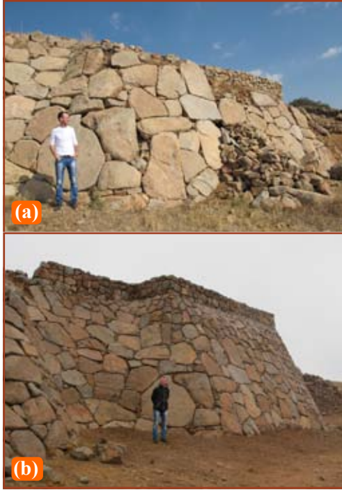
Figure 17. (a) Architect Erkan Kambek contemplating the huge task ahead. (b) With a team of five skilled masons work was completed in less than a month.
