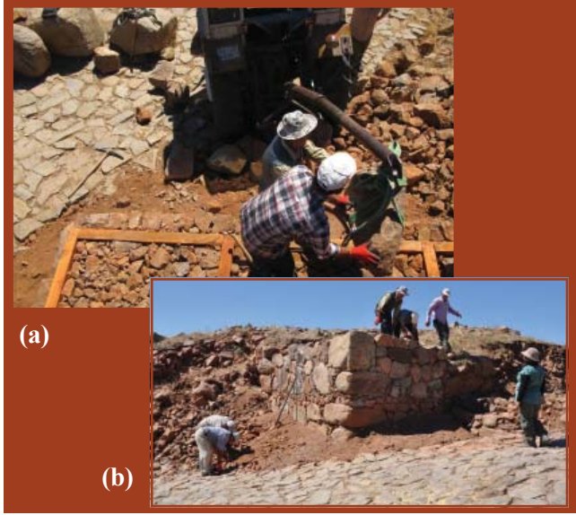
Figure 15. (a) After placing timber beams and levelling with small stones, large stones were lifted with the help of the tractor and its hydraulic lifting system. (b) Repair of the West Tower in progress.
